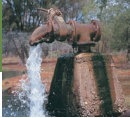
Capping of leaking bores: an imperative for groundwater management
