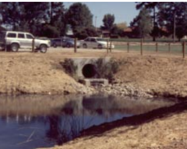
A storm water pipeline, Wareena Wetlands, Wangaratta.
