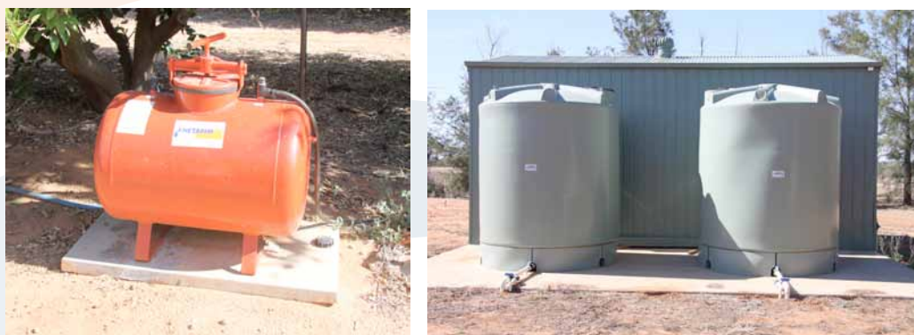
Figure 1 Examples of tanks used to dissolve fertilisers in fertigation systems
