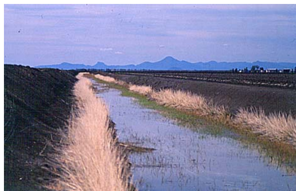
An irrigation channel heavily infested with brown beetle grass. The infestation has been sprayed with glyphosate and burned off, but will regrow.
