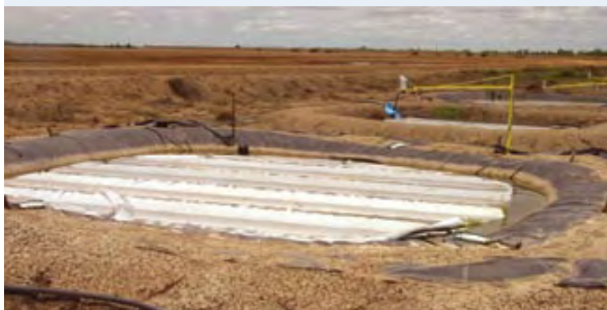
Figure 2.7.5. A dam cover fully installed, proving to be an effective method of reducing evaporation from storages
