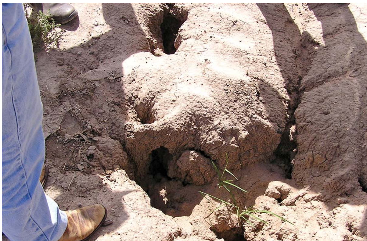
Figure 5.2 Cracking, erosion and tunnelling of embankment crest
