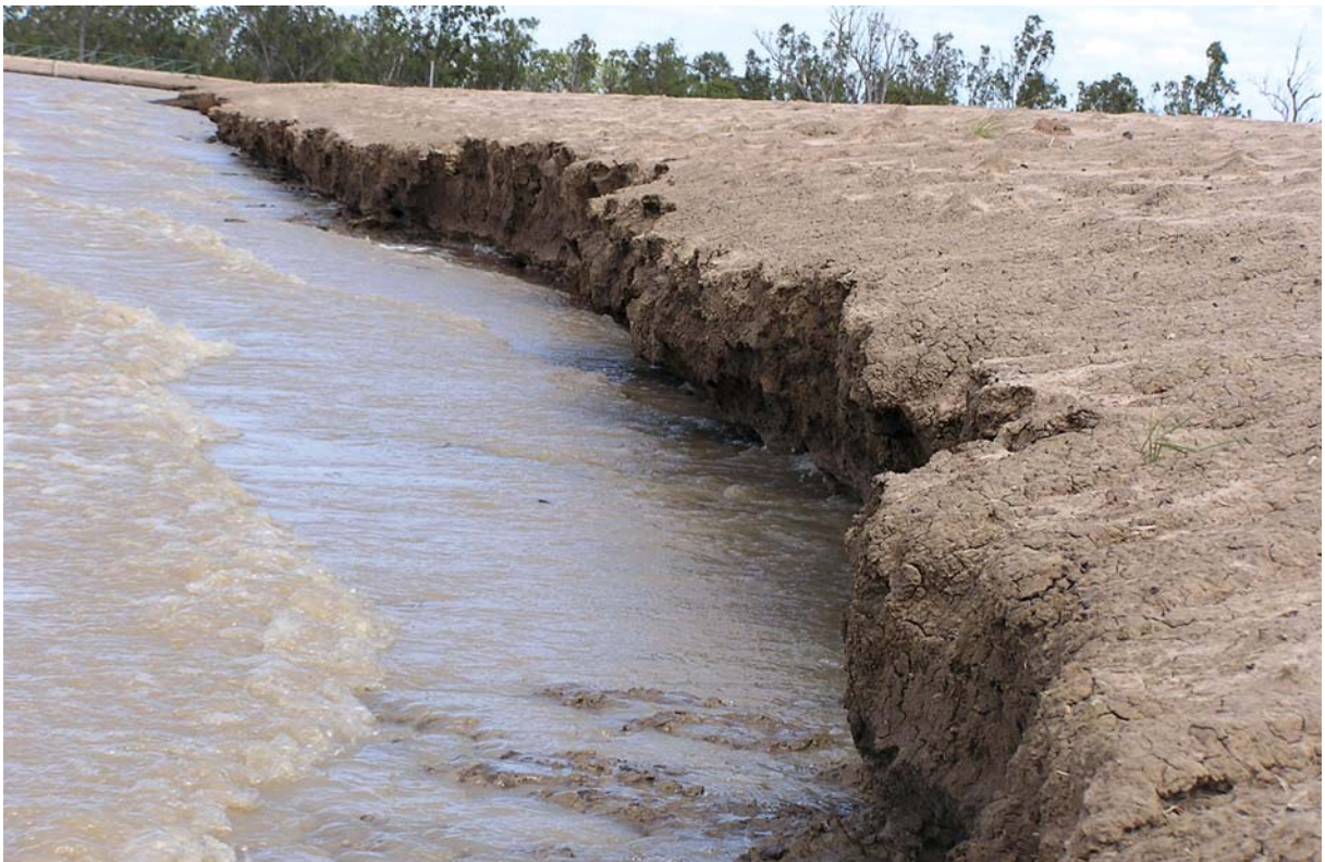
Figure 5.4 Wave erosion on the inside batter
