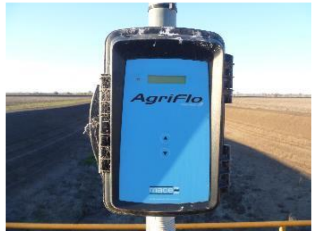
Water low and volume metering
