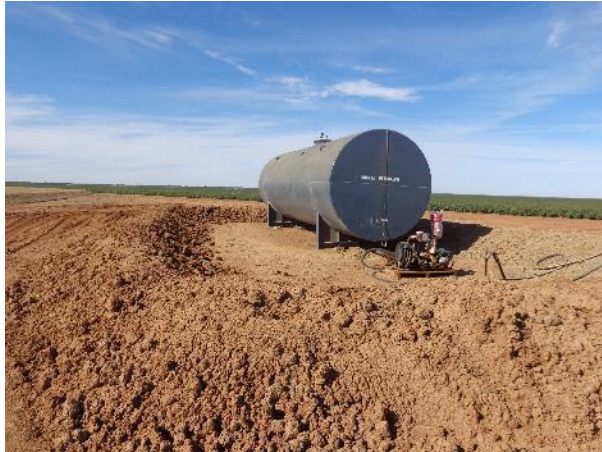
An earth bunding of a large petrochemical tank
