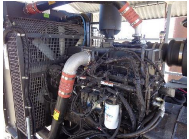
Upgrade pump motor with remote energy use monitoring
