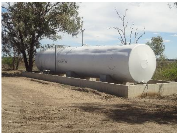
Bunded petrochemical storage
