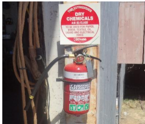
Fire extinguishers in place
