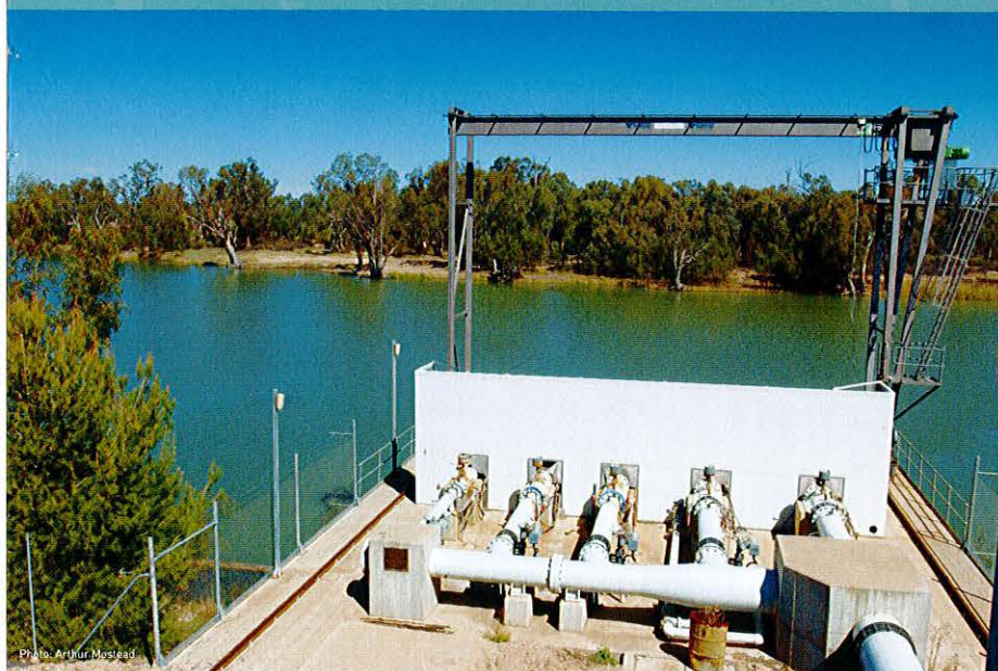
Pumping station on the Murray River at Curlwaa, New South Wales
