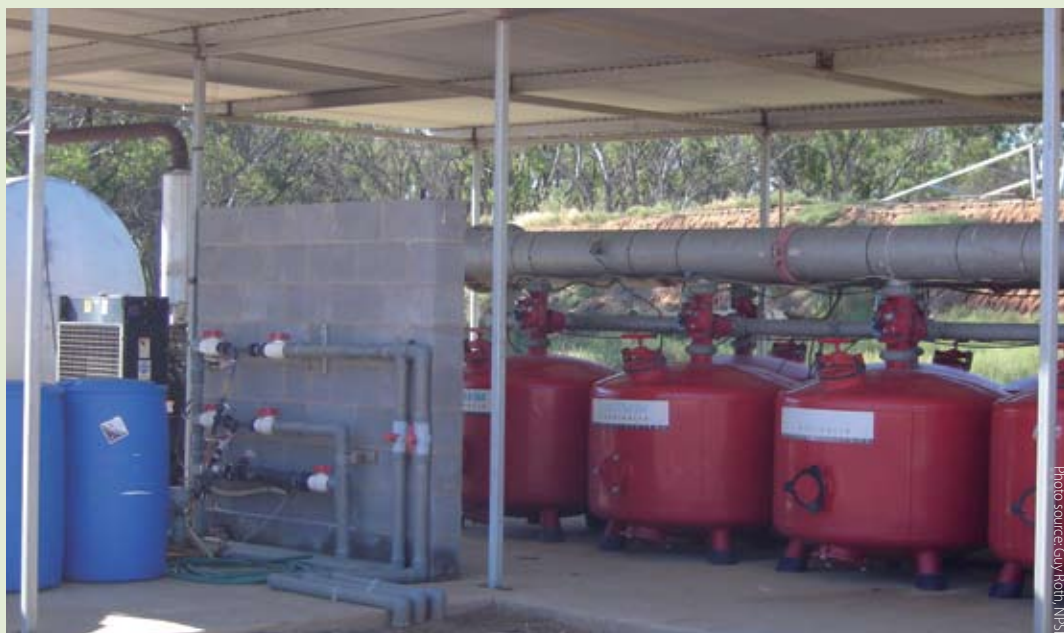
Part of Stewart's irrigation system.
