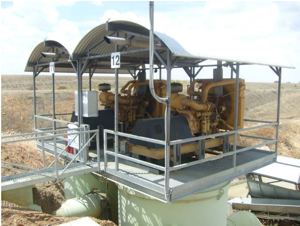
Figure 4 Pump Station on Keytah (1 of 26)
