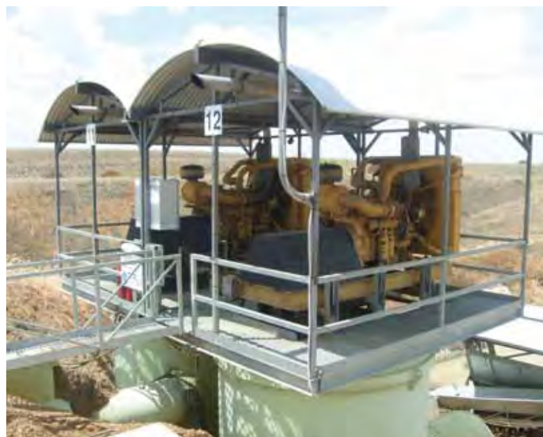
Detailed monitoring may include performance of pumping systems and stationary motors.
